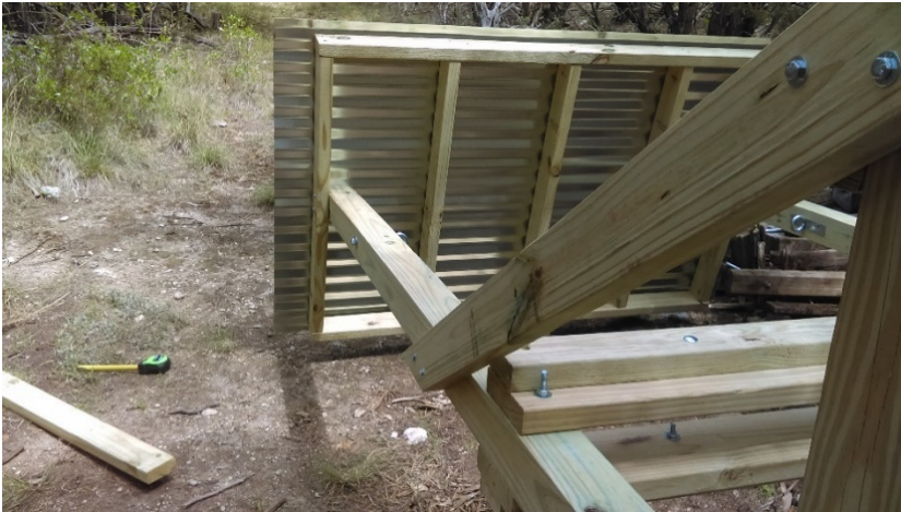
View of bottom support carriage bolts. Lag screws fastening the rear supports.
