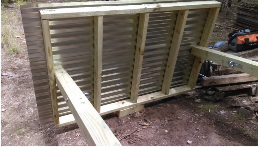
View of the 4x4 holding the roof frame. This allows for metal roof installation.
