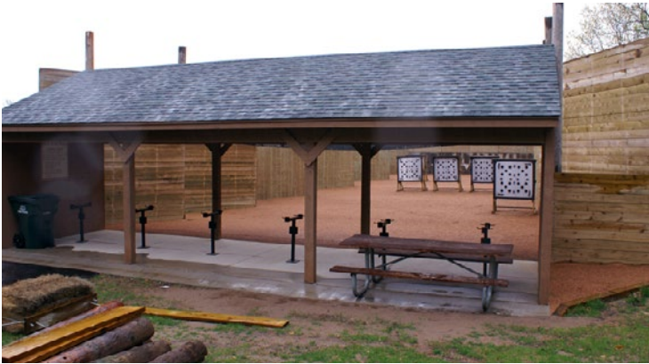
↑ Archery pavilion/containment range utilizing only ½ acre and located next to a dog park. 📍 STARING LAKE PARK , Eden Prairie, Minn.
